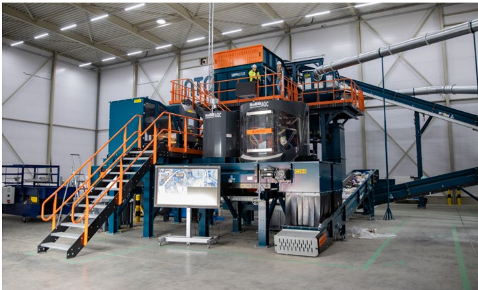
THE NEW NTCP PLANT (NETHERLANDS TESTCENTRE CIRCULAR PLASTICS)
